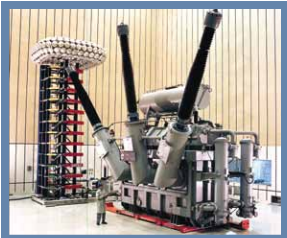
Karkhe Hydro Power Plant 160 MVA – 13.8 / 410 KV
