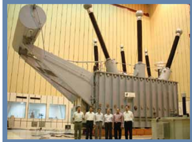
Power Transformer – Fars 315 MVA – 400 / 230 / 20 KV
