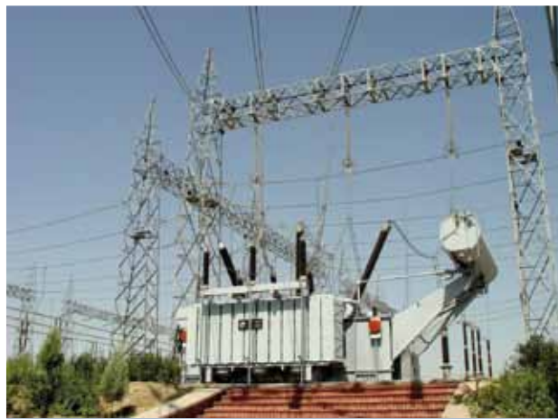
Toos Substation 200 MVA – 400 / 230 / 20 KV
