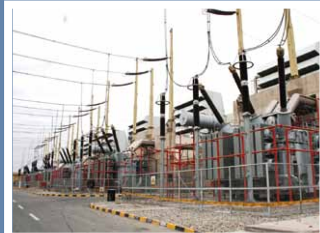
Damavand Power Plant 200 MVA – 15.7 / 420 KV
