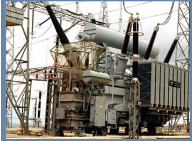
Power Transformer 200 MVA – 400 / 230 / 20KV
