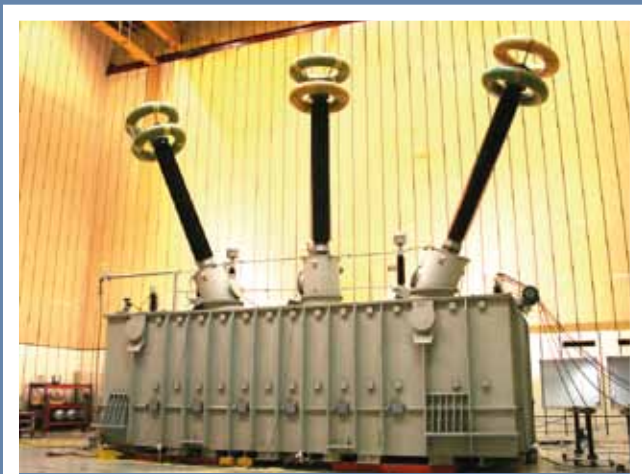
Power Transformer – Neiriz 200 MVA – 400 / 66 / 20 KV
