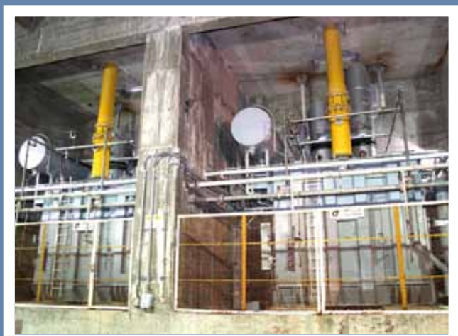
Karoon Hydro power Plant 100MVA – 15.7 / 420 KV
